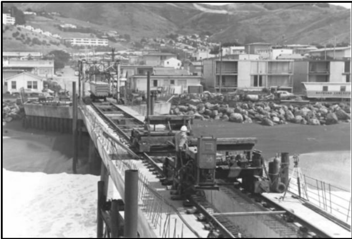
On March 20, 1973, employees of Healy Tibbitts Construction Co. of San Francisco work on the building of the City of Pacifica's Ocean Fishing Pier and Outfall. (Photo courtesy of the Pacifica Historical Society.)
