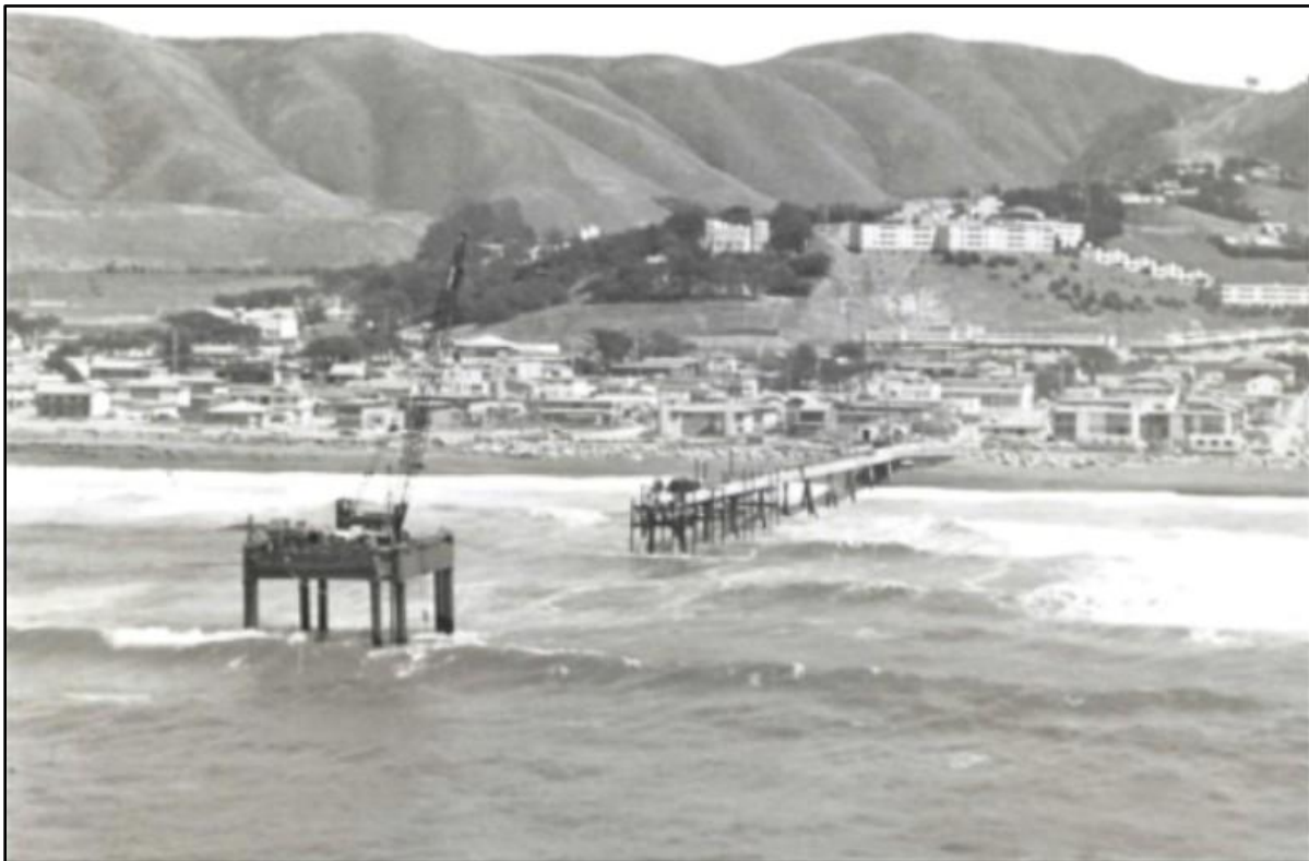
This Pacifica Pier in-progress photo was taken on April 20, 1973. Workers were flown in by helicopter because a helicopter took 5 minutes to deliver the construction crew, whereas a boat on a heavy sea could delay the work, each way, by anywhere from 30 to 45 minutes. (Photo courtesy of the Pacifica Historical Society.)
